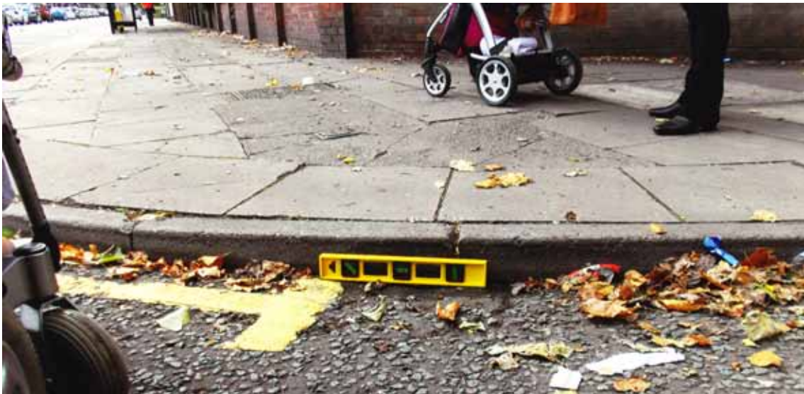
Albany Rd Derby Lane left side
